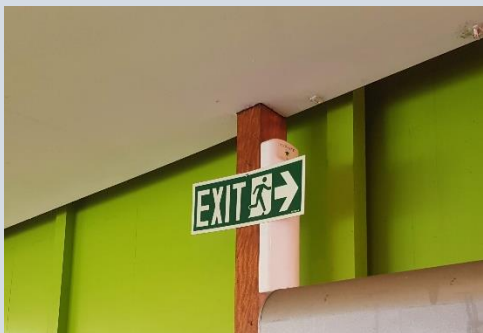
An installation without a dedicated light source and the required emergency light
