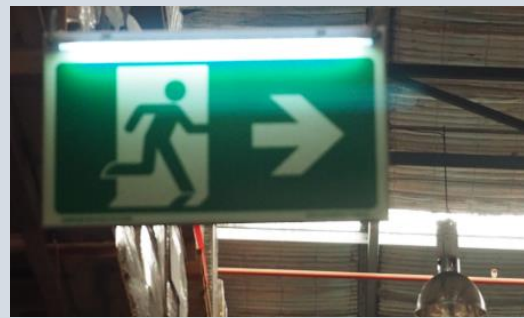
Strip lighting doesn't illuminate whole surface with 100 lux
