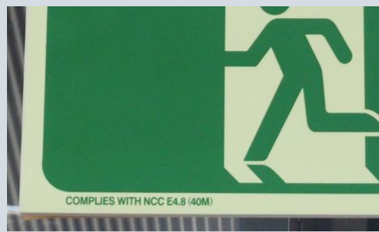
Rated distance of 40 m is non-compliant to AS/NZS 2293.1 (maximum 24 m)
