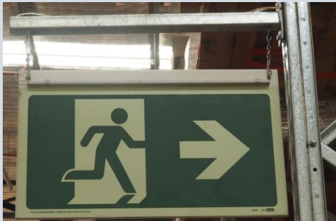
Strip lighting has failed making the sign non-compliant
