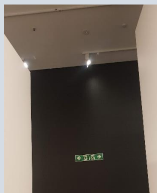
Track lights may be moved from their original positioning, making systems non-compliant
